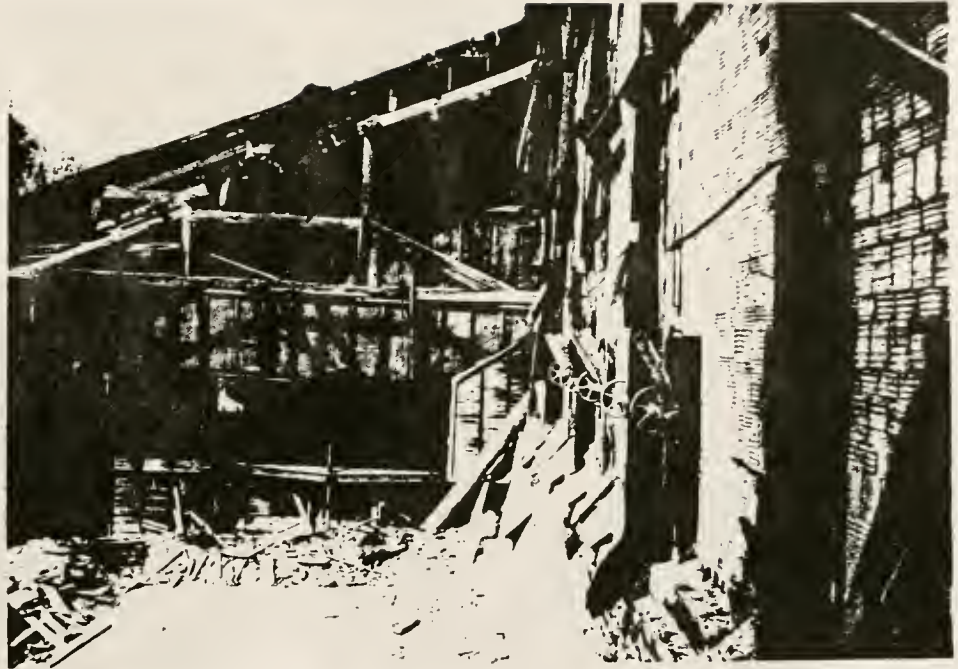
Figure 158. Arsenic plant (structure #59) showing area containing McDougall roasting furnace (arrow) and discharge gates (arrow) for emptying the primary kitchen along right, north view.
